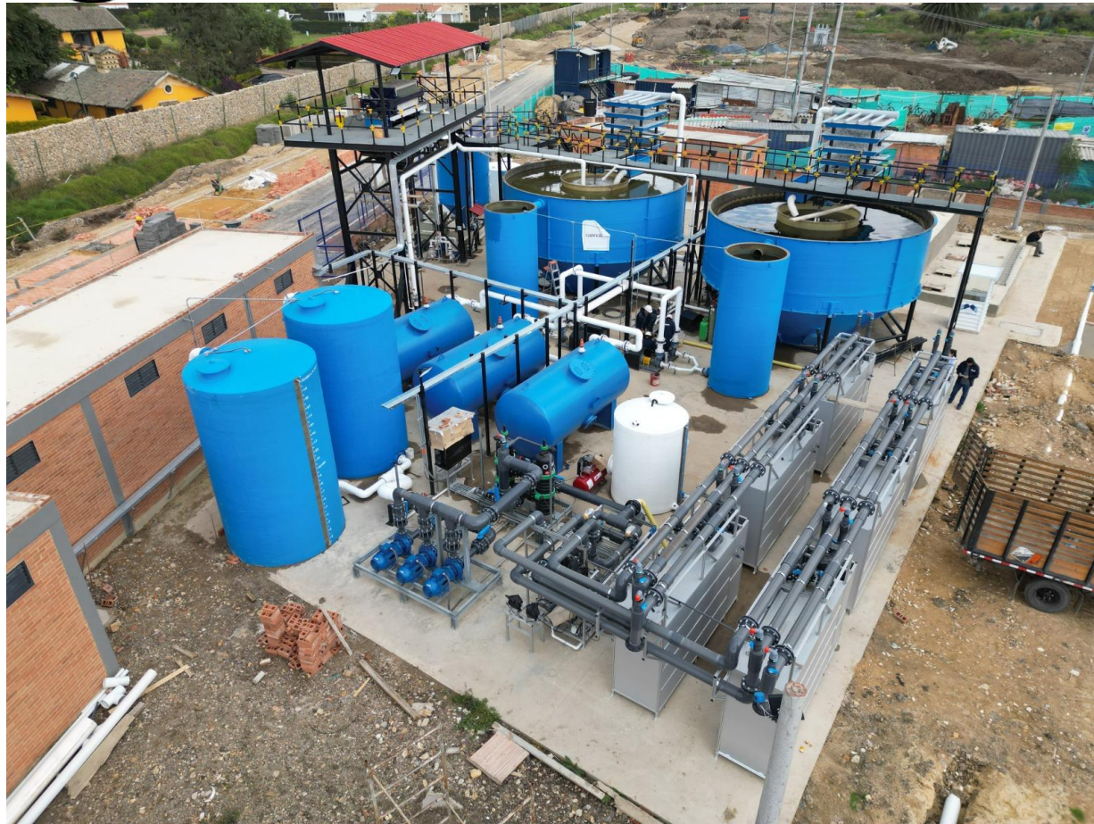
Drinking water purification System – 240 m 3 /h - Colombia
