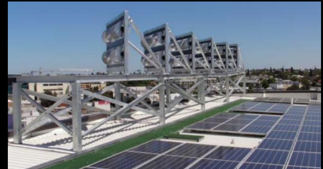
Combine wind and PV on one rooftop
