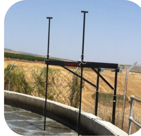
K'far Tabor DWWTP (AS) Q=500 cubic meters per a day
