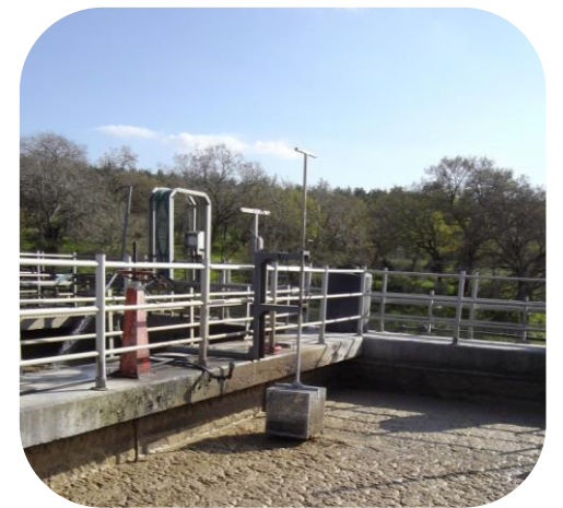
Ha-Solelim DWWTP (MBR) Q=2400 cubic meters per a day
