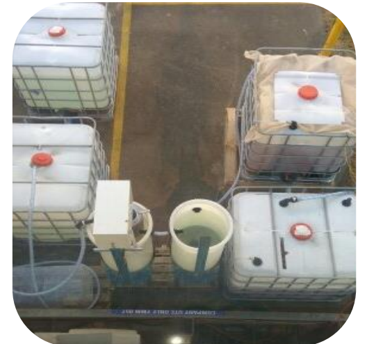
Winery wastewater treatment Q=150 cubic meters per a year
